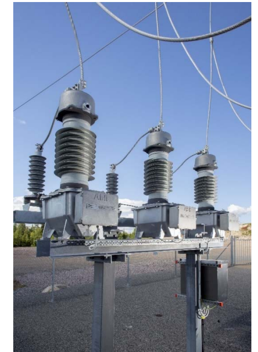
Plate 5.16 - Typical Voltage Transformer Image: ©ABB
