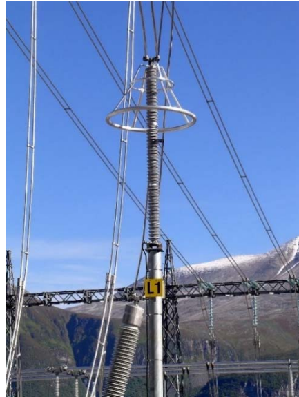
Plate 5.7 – Typical HV Surge Arresters Image: ©ABB
