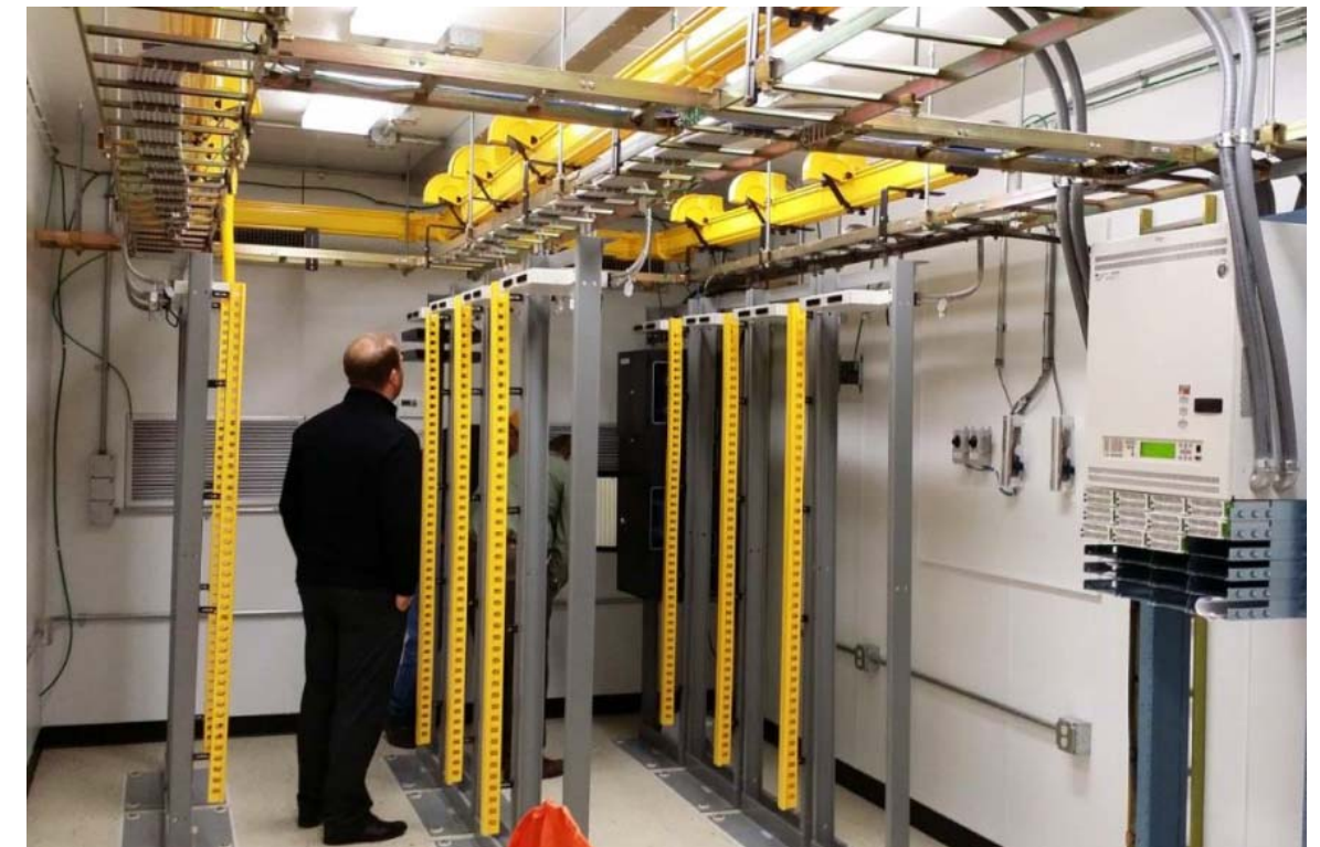
Plate 5.39 – Indicative illustration of an ORS Building (Copyright – B&M FOC Review Report Issue D Sept. 2018)
