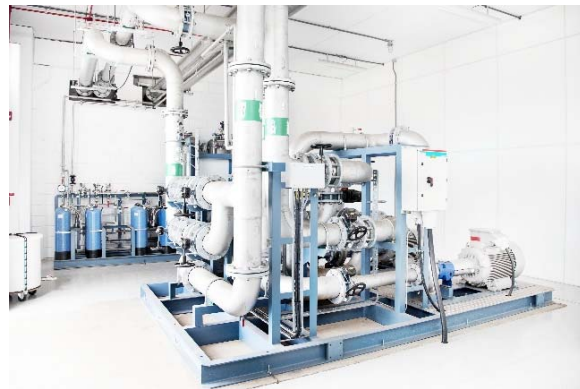
Plate 5.22 – Typical Water Pumping Station Image: ©ABB
